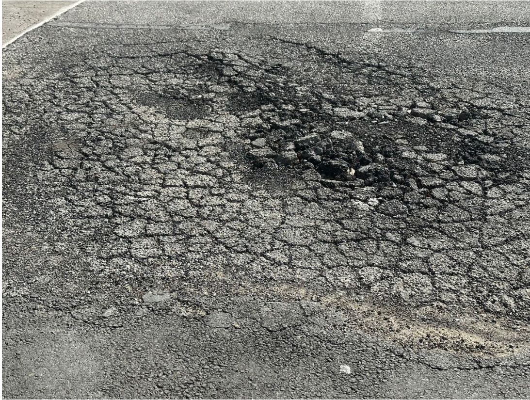
Photos of bad sections of parking lot
