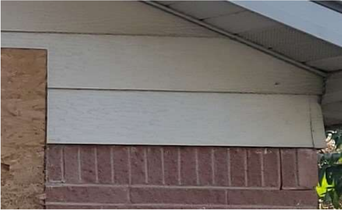
White putty (3% Chrysotile) on insulation behind aluminum siding
