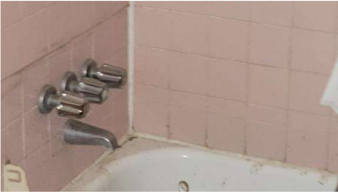
Caulking around tub
