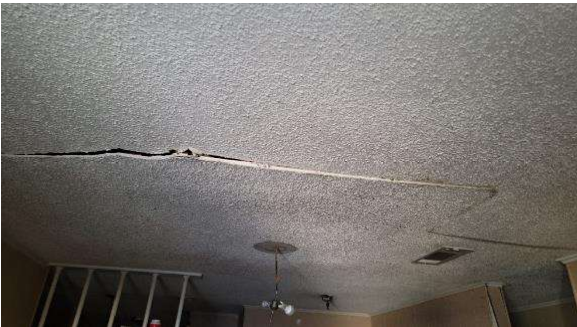
Ceiling texture (joint compound 2% Chrysotile)
